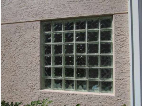
unprotected glass block
